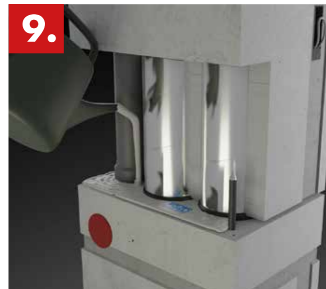
9. Connect the units by applying grouting concrete to the interface between them.
